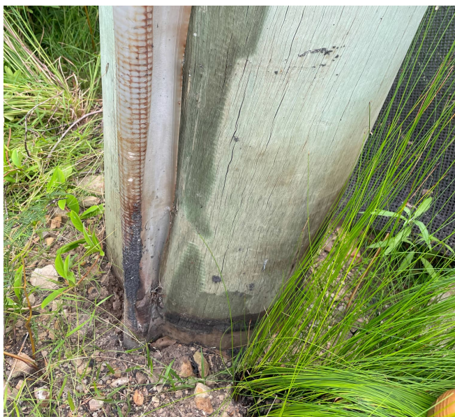
Figure 4 – Impacted transmission pole after Fire Mesh.
