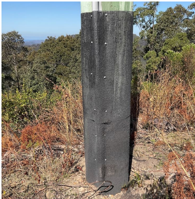
Figure 3 – Transmission pole impacted by grass fire.
