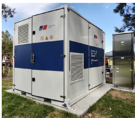
Photo: Rolls Royce 'MTU' 445kWh up to 200kVA output
