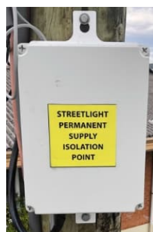
Photo 2: LV/SL isolation box
