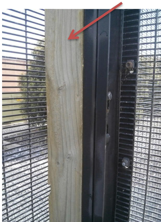
Correct substation isolation but no danger sign
