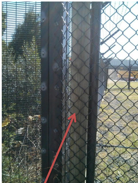
Compromised isolation – Metallic connection across isolation point
