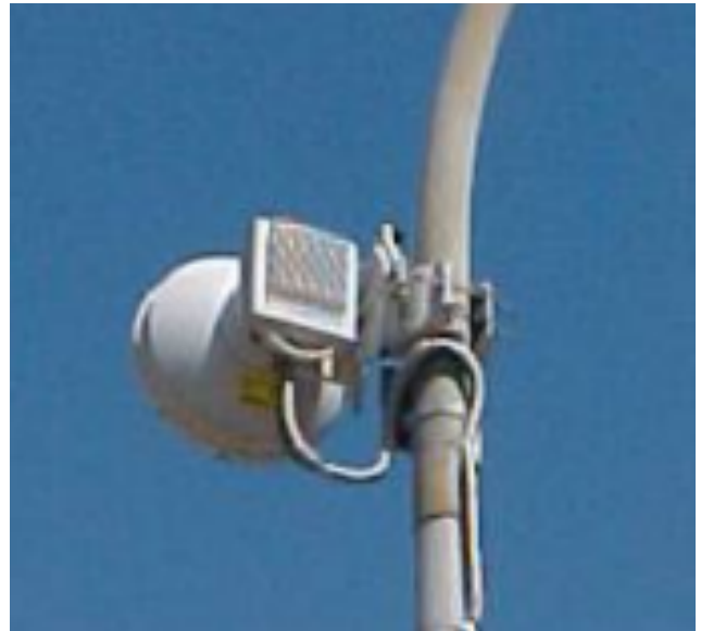
Parabolic Dish type antenna
