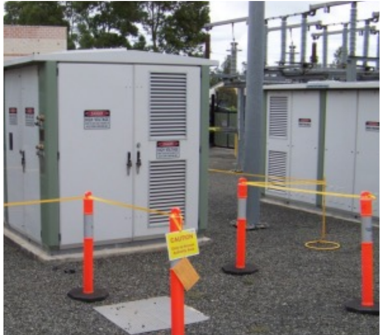
Figure 13 – Barrier “in” method for the erection of a barrier in a substation
