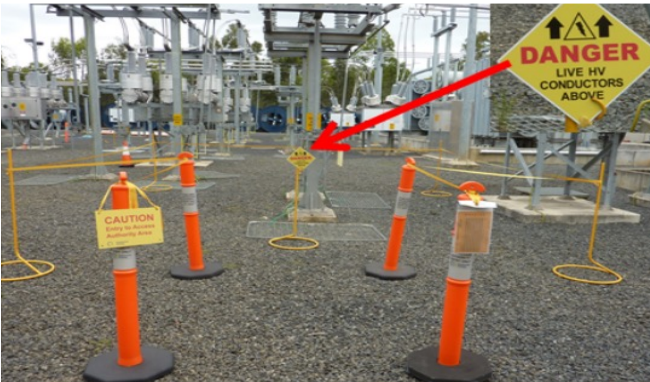
Figure 12 – Barrier “in” method for the erection of a barrier in a substation showing “DANGER live HV conductors above”
