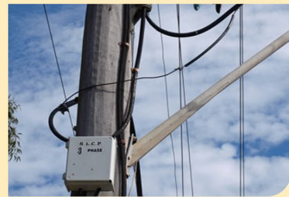
Figure 18 – Example of pilot cable
