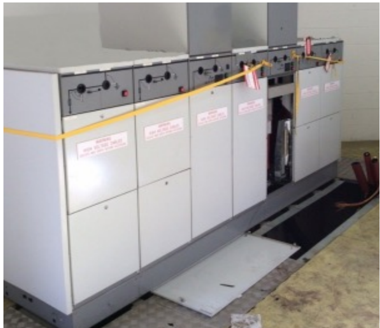
Figure 14 – “Barrier “out” method for the erection of a barrier on totally enclosed switchgear
