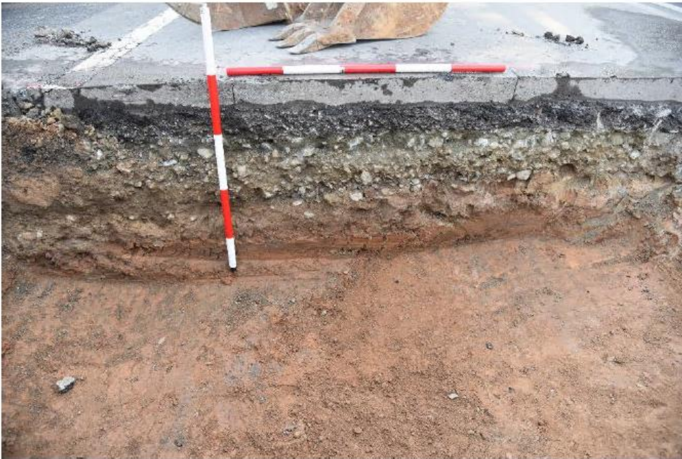
Figure 9-2 Section of trench dug through a similar road in Prospect showing evidence of disturbance to a depth greater than 30 cm (Source: Artefact 2022a; Artefact 2019b).
